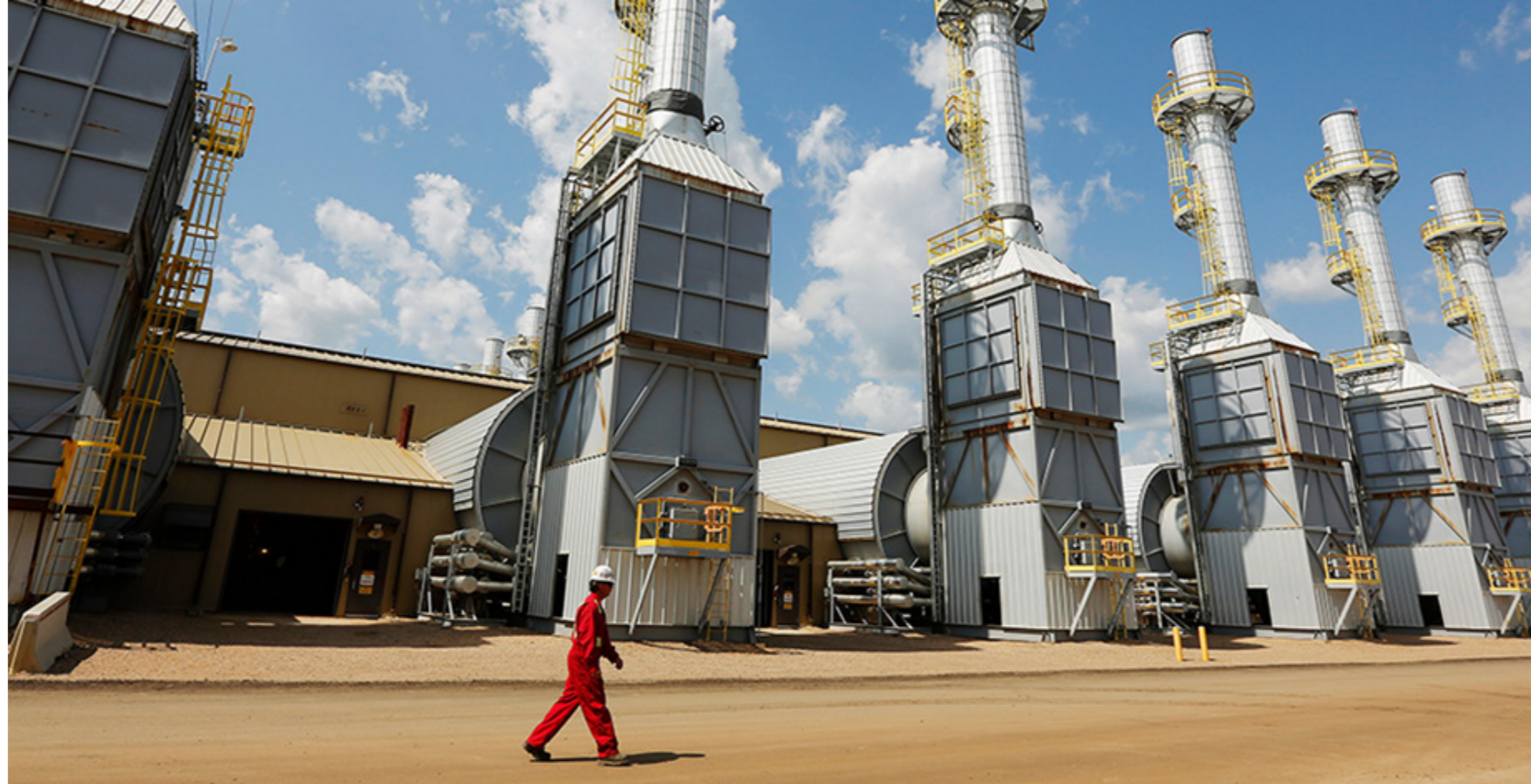
The steam generating facility at the Cenovus Foster Creek SAGD oil sands operations near Cold Lake, Alberta
